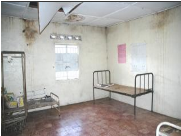
A ward at the Barmoi clinic in desperate need of renovation
